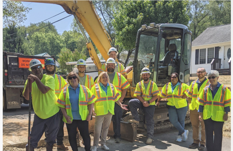
VRSA underwriting, member services, and risk services staff attended a sewer lateral repair being performed by staff of the Western Virginia Water Authority.
